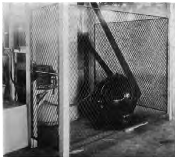
Fig. 3. Isolation or Enclosure of Motor located in Work-Room.†
